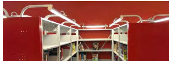
LED AISLE LIGHTING
